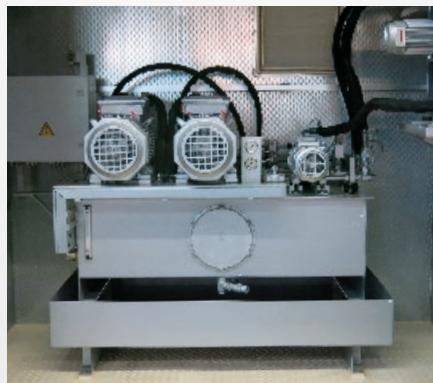
Lime shaft pre-heating
